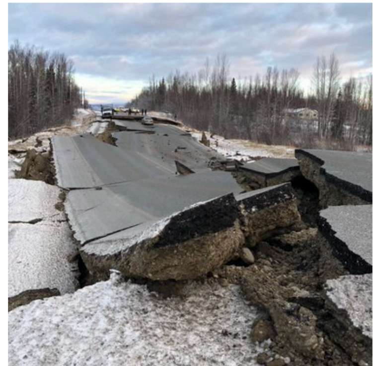
Images from the aftermath of the Anchorage earthquake
